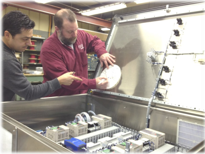
Above: Scot Shepard EB Controls supervisor shown testing out PLC logic as part of the thorough 15 point quality inspection process.
